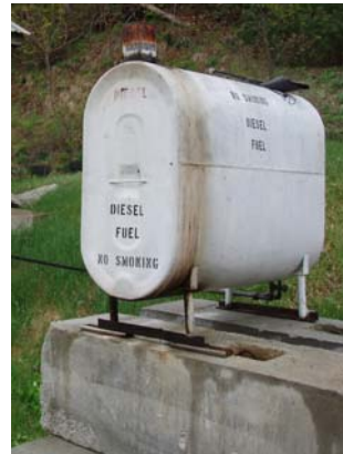
Improper containment note drips
